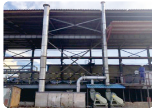
Completed installation of acid mist fan
