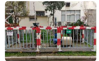
Upgrade and replacement of interceptor valves of rainwater interception pools for Quzhou Huayou
