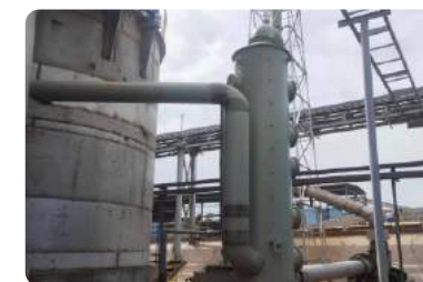
Acid mist absorption device in leaching tank of wet process plant in Africa MIKAS
