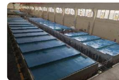
Desalination treatment plant of high salinity wastewater in Huajin
